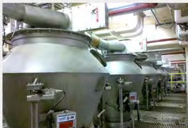
6" (152mm) Fill Pass Diverter above a scale hopper handling baking mixtures
