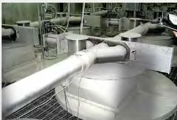
5" (127mm) Fill Pass Diverter above a scale hopper handling calcium carbonate
