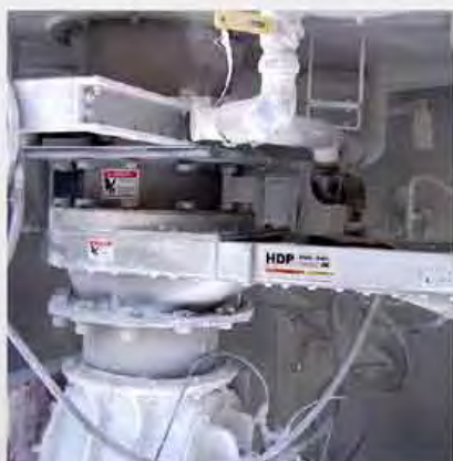
16" (406mm) HDP above airlock handling calcium oxide
