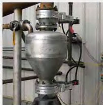
12" (305mm) HDP above and below a pressure pot handling PRB coal and wood chips
